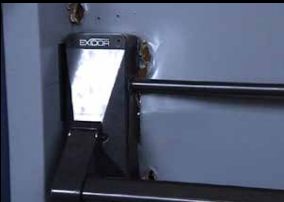
Inside view after 10 mins and the 4th bolt is still holding the door secure.
